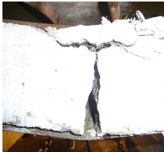
Figure 6. Crack at mid span of Profile sheet slab
