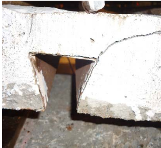
Figure 5. Crack Pattern of Re-entrant Profile sheet slab
